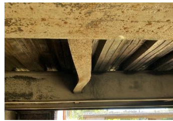
Fig. 2. Buckled Lateral Member
