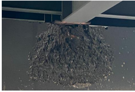
Fig. 3. Spalling at Top of Pier
